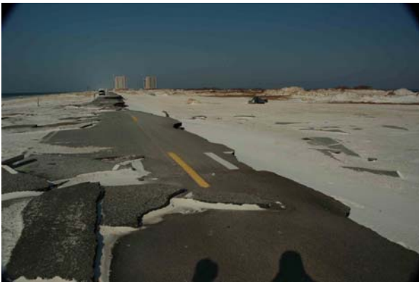
Photograph Q. Pavement damage to FL 399 east of Pensacola Beach.
