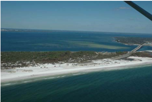
Photograph S. Repairs underway on US 98 west of the East Pass Bridge.
