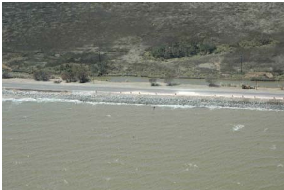
Photograph A. AL 193 revetment damage repairs. This damage was partly due to inadequate rock sizes for the storm waves.
