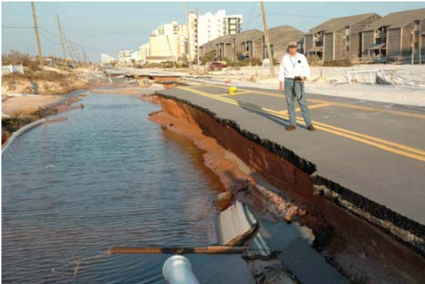
Photograph G. Pavement damage on north side of FL 292 due to "weir-like" flow down back side.
