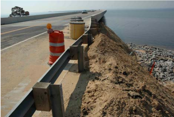
Photograph P. Repairs to damage at north end of Garcon Point Bridge
