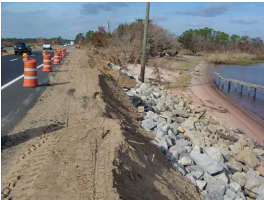
Photograph L. Repairs to damages to US 90 at north end of Escambia Bay arm of Pensacola Bay. Numerical simulations indicate that this end of the bay should have had the highest surge elevations and very large wave heights (up to 9 feet). The existing shore protection was not adequate to protect the road.
