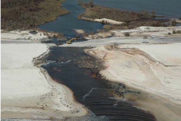
Photograph F. Ongoing repairs to breach in AL 182 at Shelby Lakes area.
