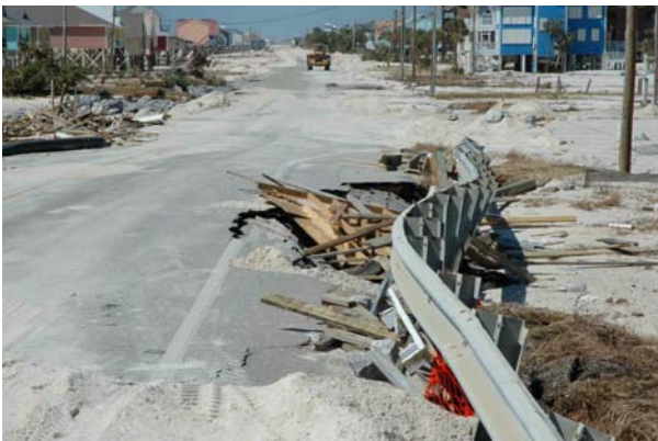
Photograph E. AL 182 emergency repairs to damage to approach to Little Lagoon bridge.
