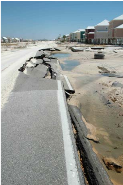
Photograph D. Pavement damage to AL 182 that was likely due to storm surge return flow.
