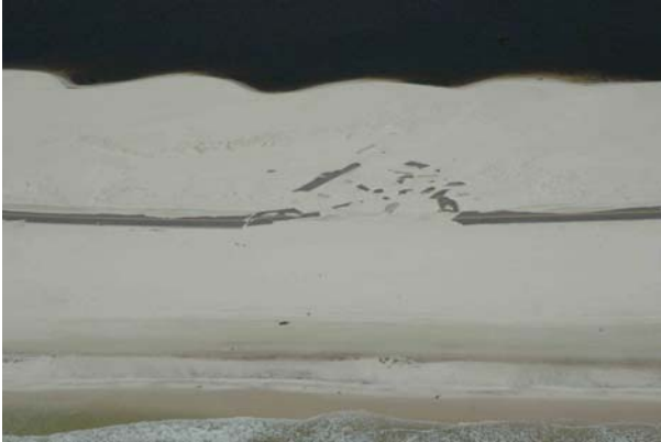
Photograph H. Pavement damage in Johnson Beach unit of Gulf Island National Seashore
