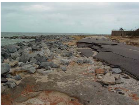
Photograph C. Pavement damage at eastern end of Dauphin Island, Alabama
