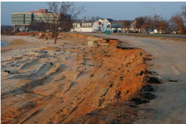
Photograph K. US 98 pavement damage in Pensacola
