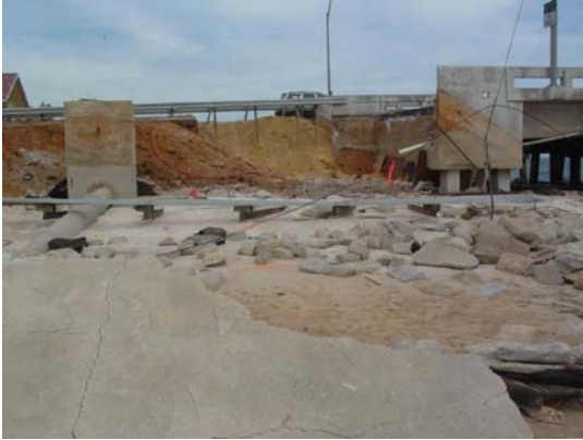
Photograph N. Damage to the approach to the bridge abutment at the north end of Bob Sykes Bridge on FL 399. Note that the entire two southbound lanes are destroyed for about twenty feet.
