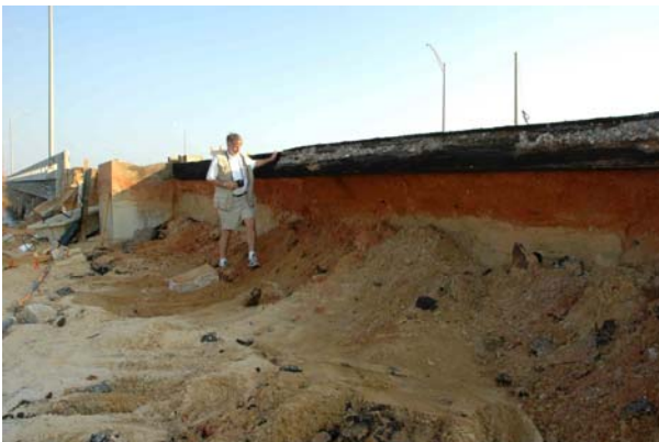
Photograph O. Wave damage to pavement on the approach at the south end of Bob Sykes Bridge, FL 399 in Pensacola Beach
